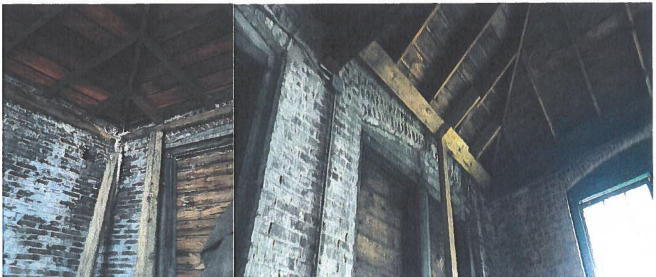
Rotted roof planks and rafters
