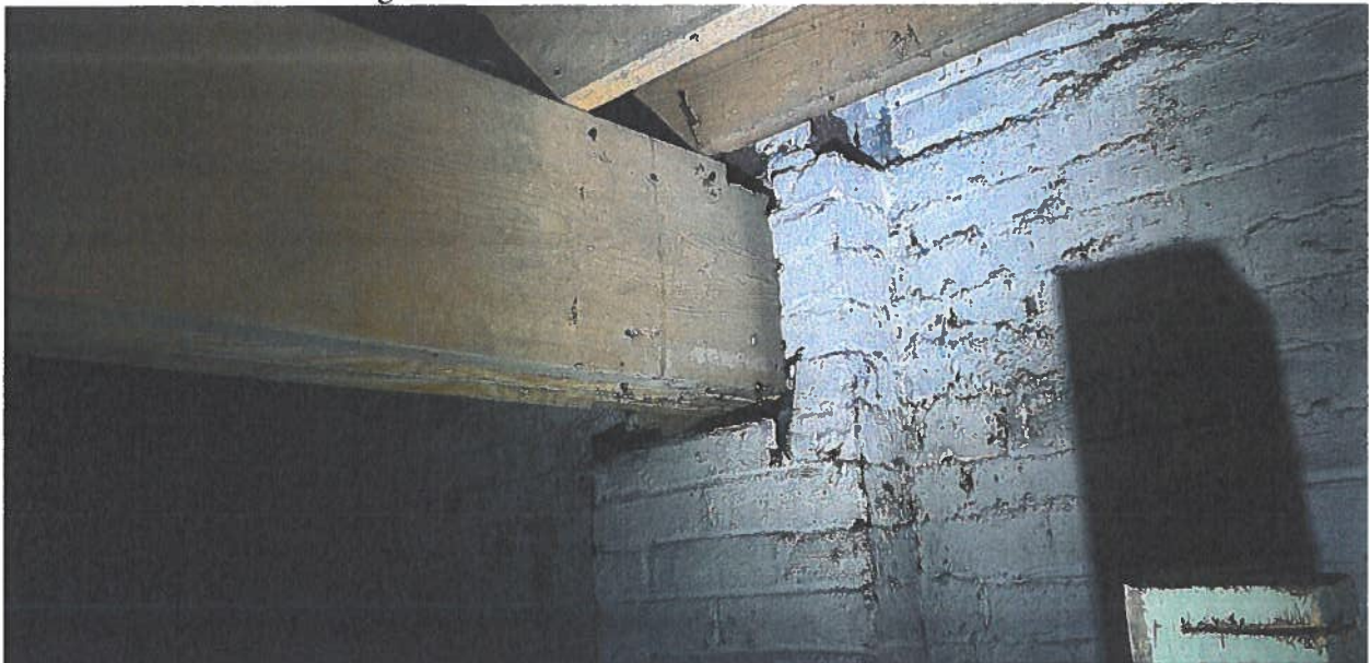
Brick column with prior repairs
