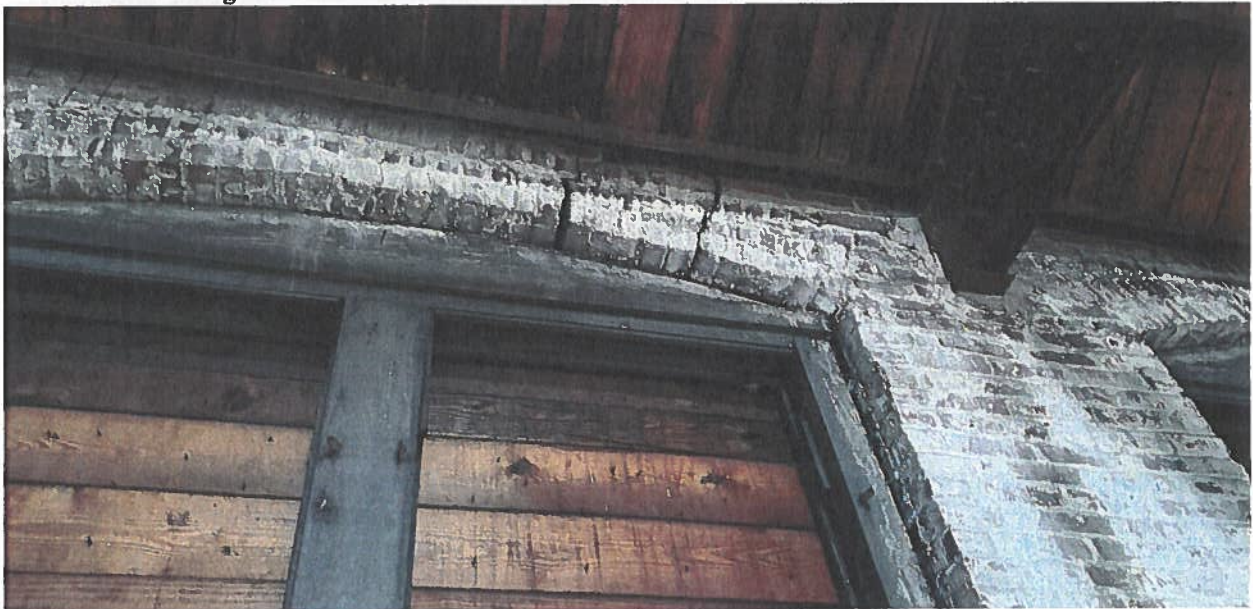
Brick arch failing
