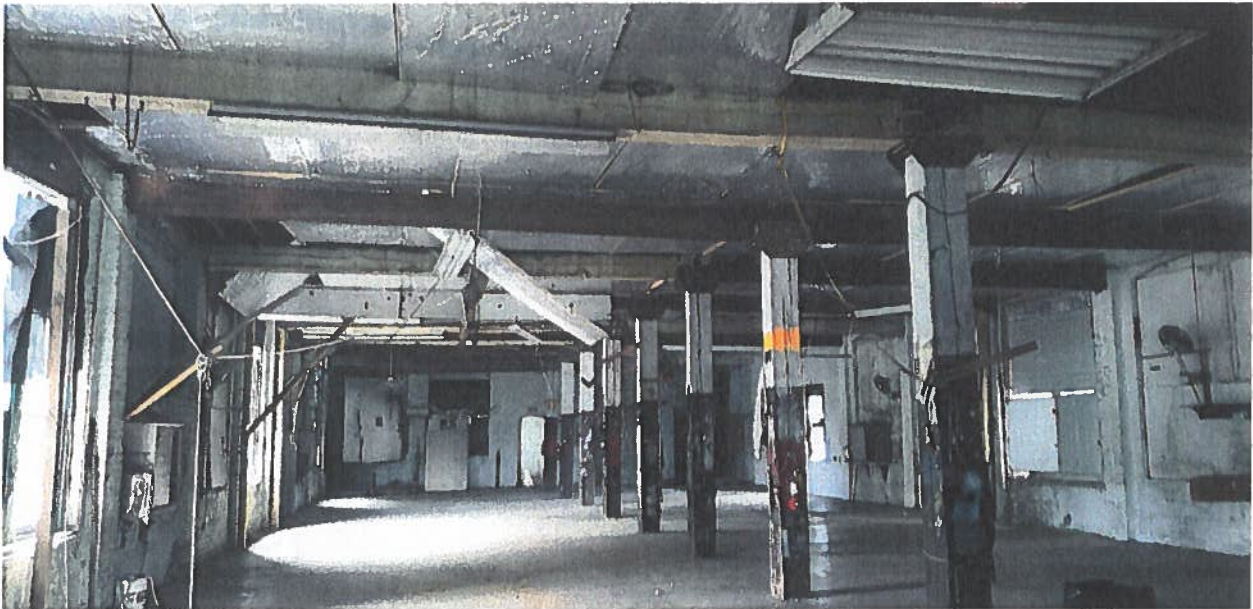
Center wood columns with cracks
