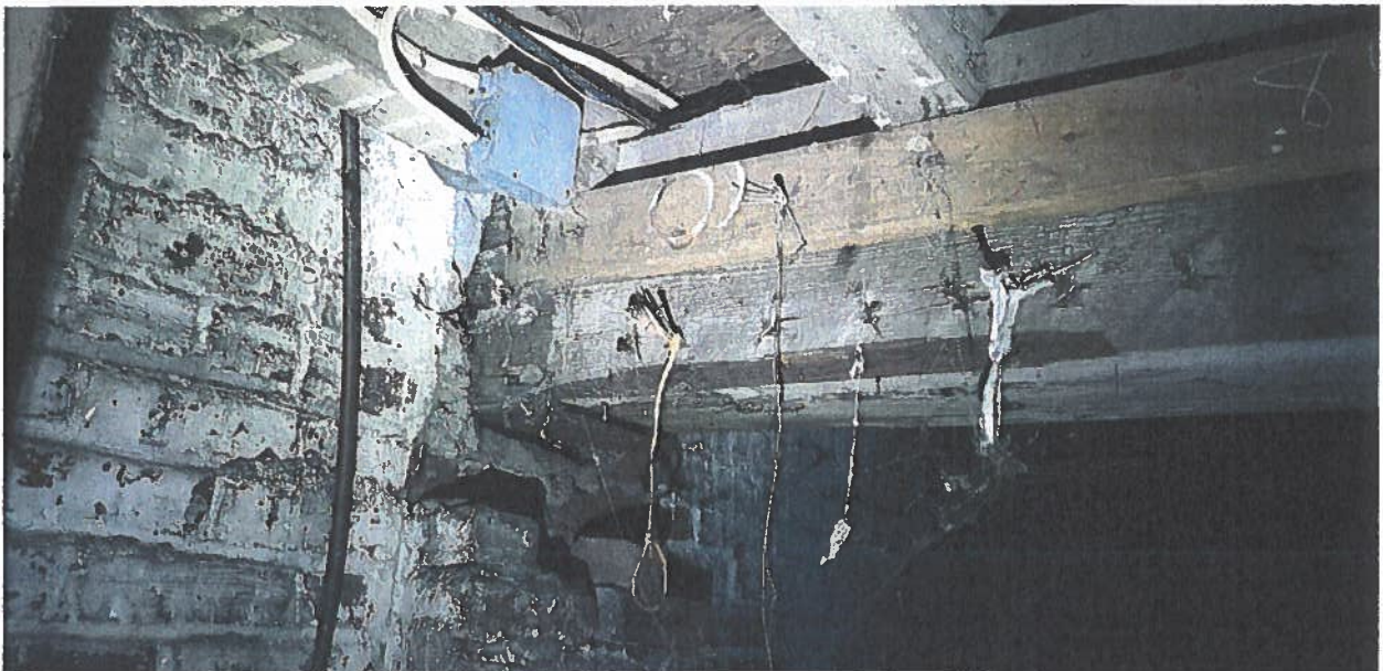
Brick column failing
