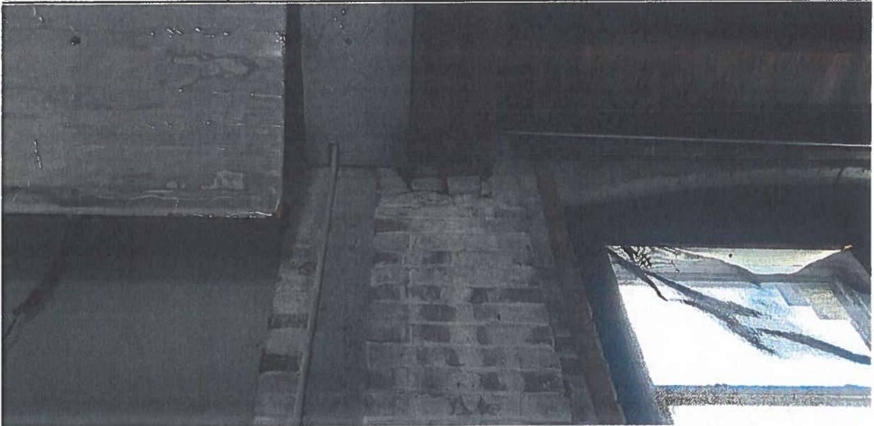
Brick column failing
