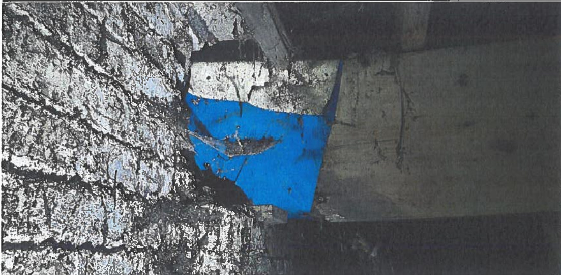
Brick column and rotted beam
