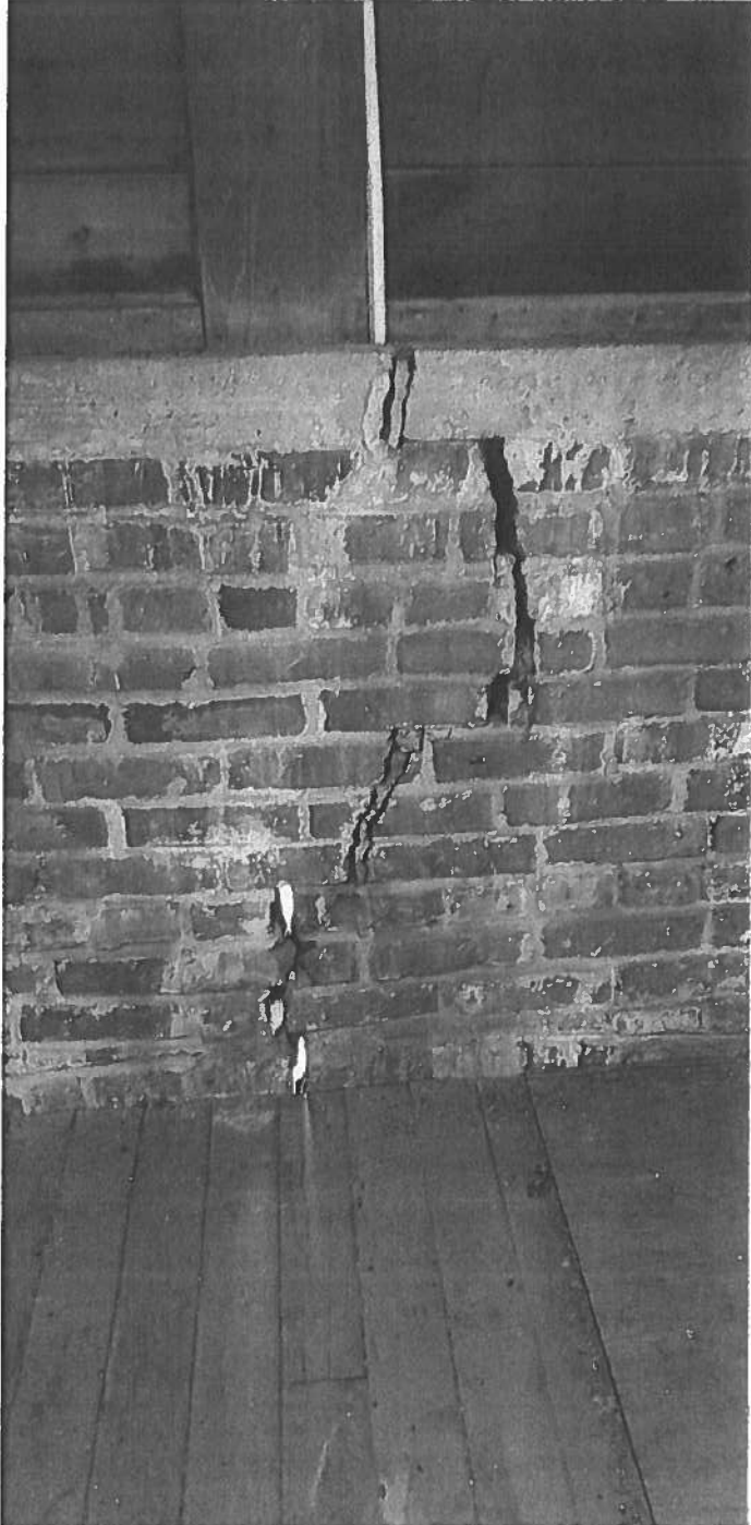
Exterior brick wall failure
