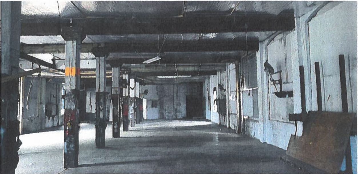
Center wood columns with cracks
